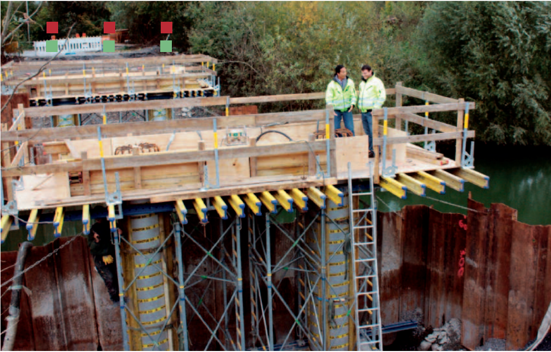
The concrete team, as a rare exception on a building site together: Cong Minh Tran and Tayyar Uysal.
